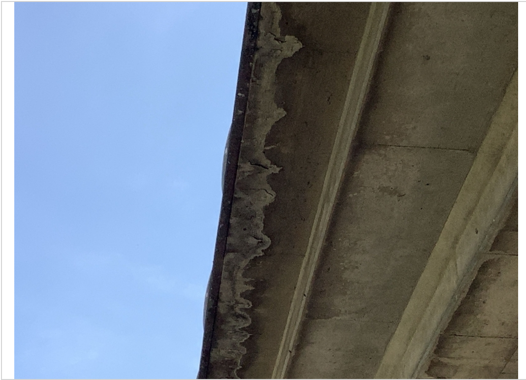
Typical delaminated areas in overhang
