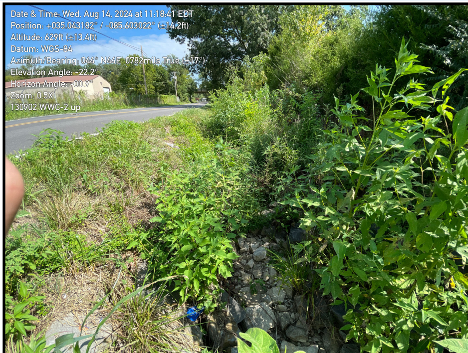
TH001746: WWC-1 *(130900.00-WWC-2) facing downgradient at inlet.
