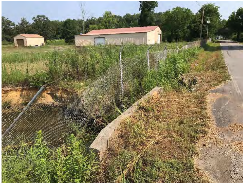
Drainage feature on Shellmound Rd
