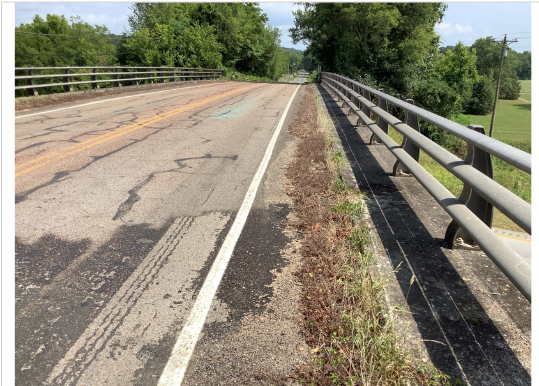
Debris on top of deck
