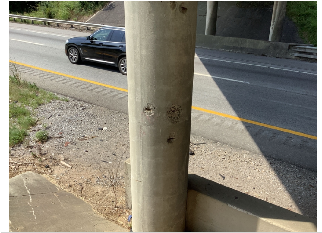
Typical spall on bents
